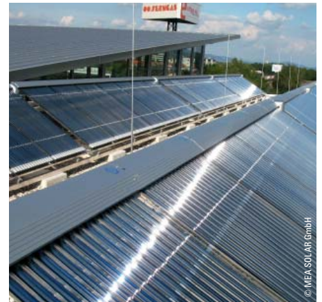
Solare Kühlung in Haid.
